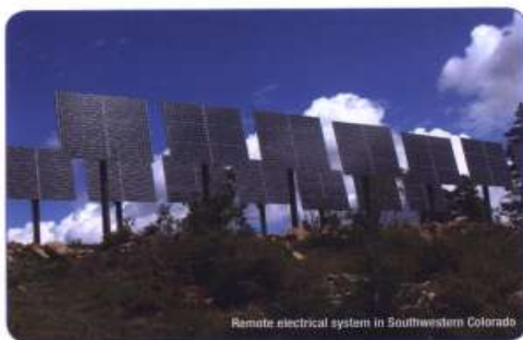
Remote electrical system in Southwestern Colorado
