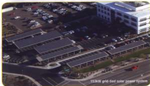
153kW grid-tied solar power system
